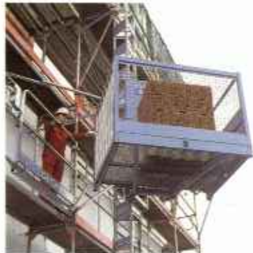
Rack and pinion hoists with steel mast
