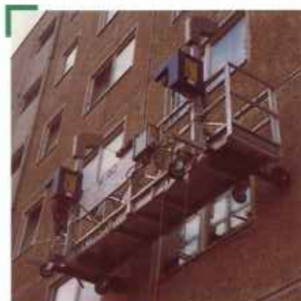
For the refurbishment of concrete facades the suspended working platforms are superior to other possibilities due to the considerably reduced setting-up time and low operating costs.
