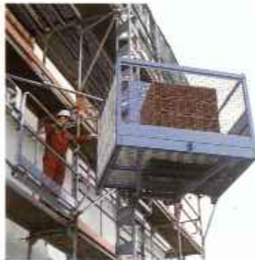
Rack and pinion hoists with steel mast
